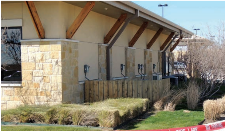
Screened HVAC units.
